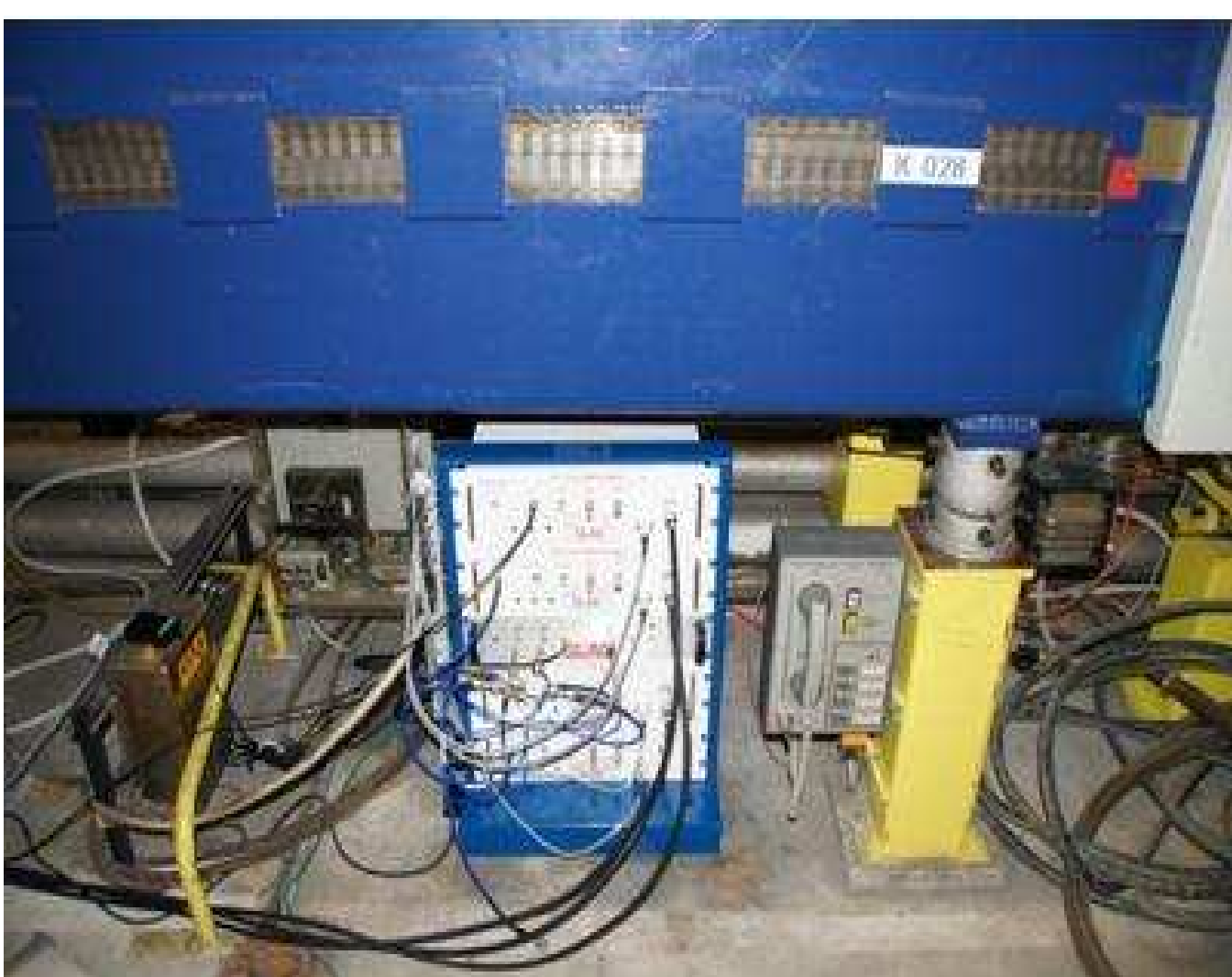
Figure 6: Four 100W amplifiers are placed in the tunnel under a bend magnet.
